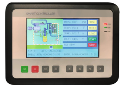
LK series System Management Control Panel
